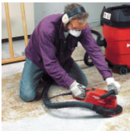
Efficient removal of remains of coatings and tile adhesives on floors or balconies
